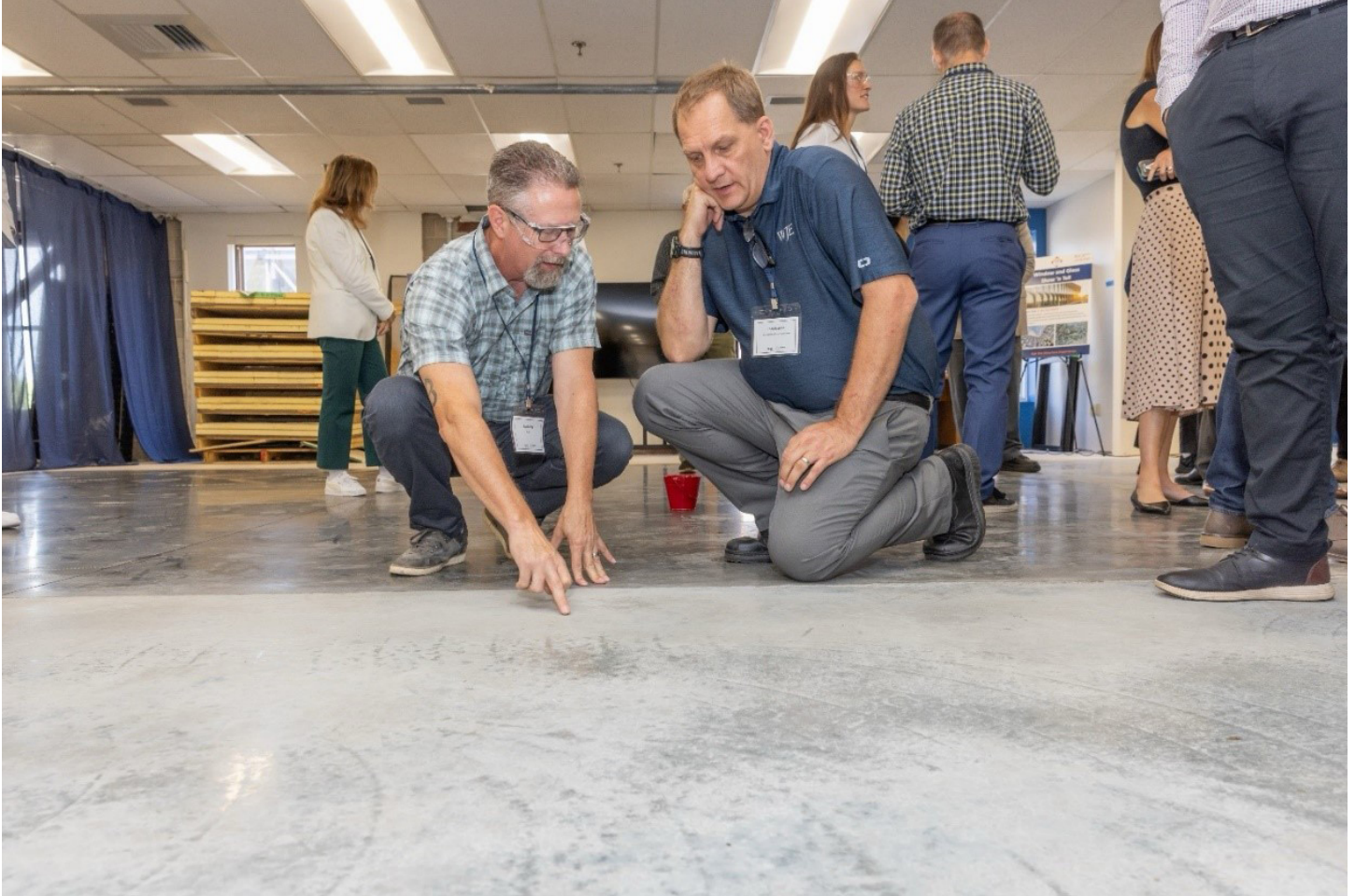
Todd Nelson from WJE (right) discussing the slab surface with Scott Kelly from Ozinga, who supplied the concrete. Final slab coloring became a constant light grey.
